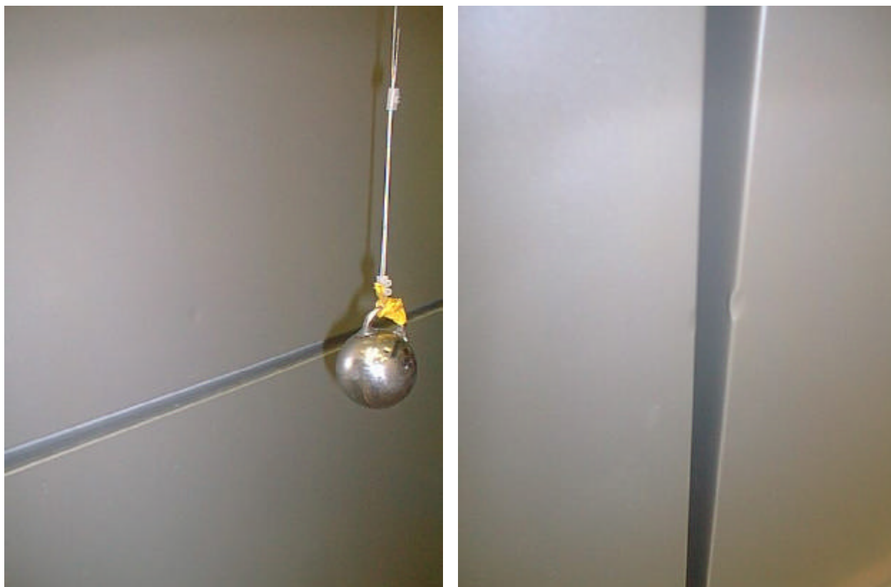
Figure A3 and A4. Showing a hard body impactor and the light indentations caused by the impacts
